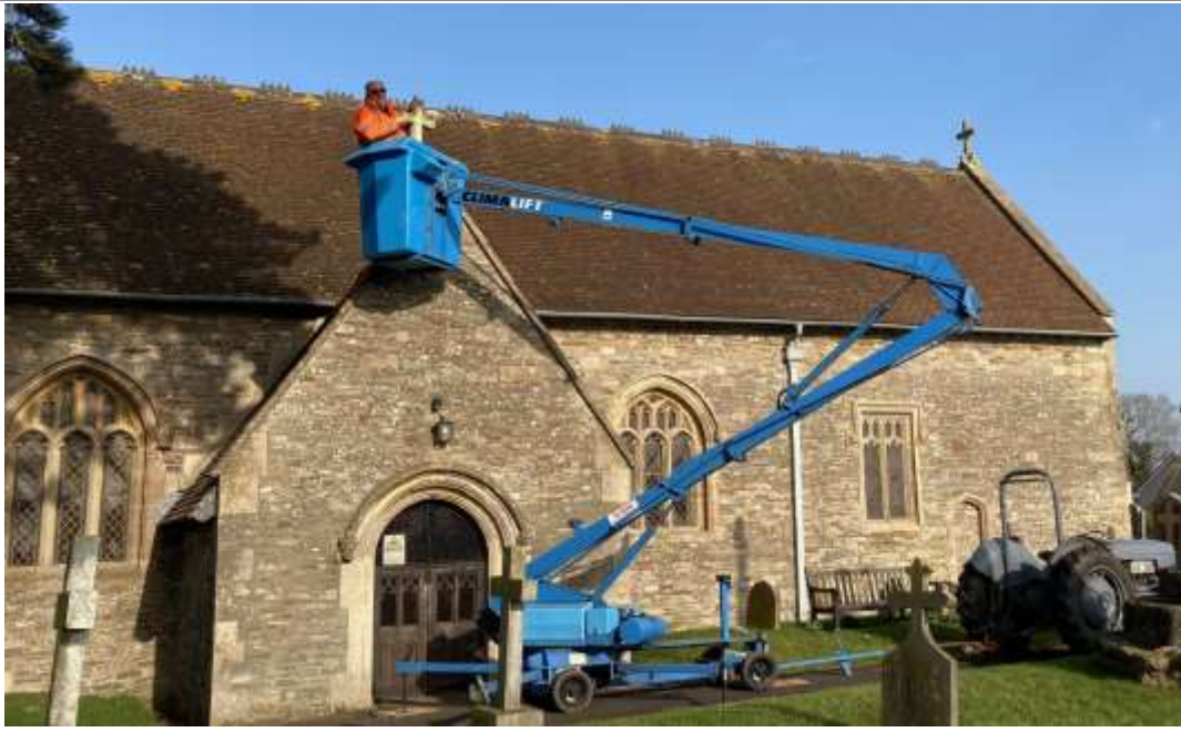
John, with Fergie and Cherry Picker removes the cross from the church porch for repair
